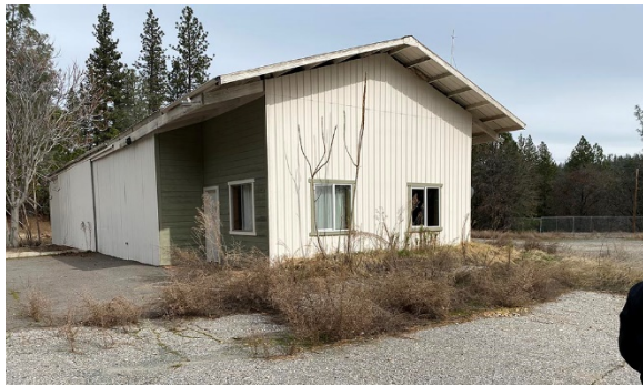
FIGURE 9 - 2ND BUILDING NOT SECURED
