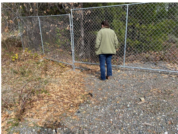
FIGURE 4 - LARGE 2+ FT GAPS UNDER THE FENCE
