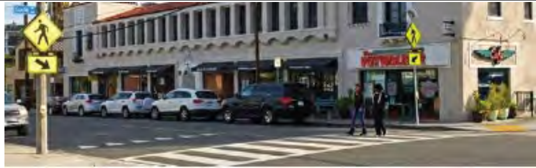
Rectangular Rapid Flashing Beacon
