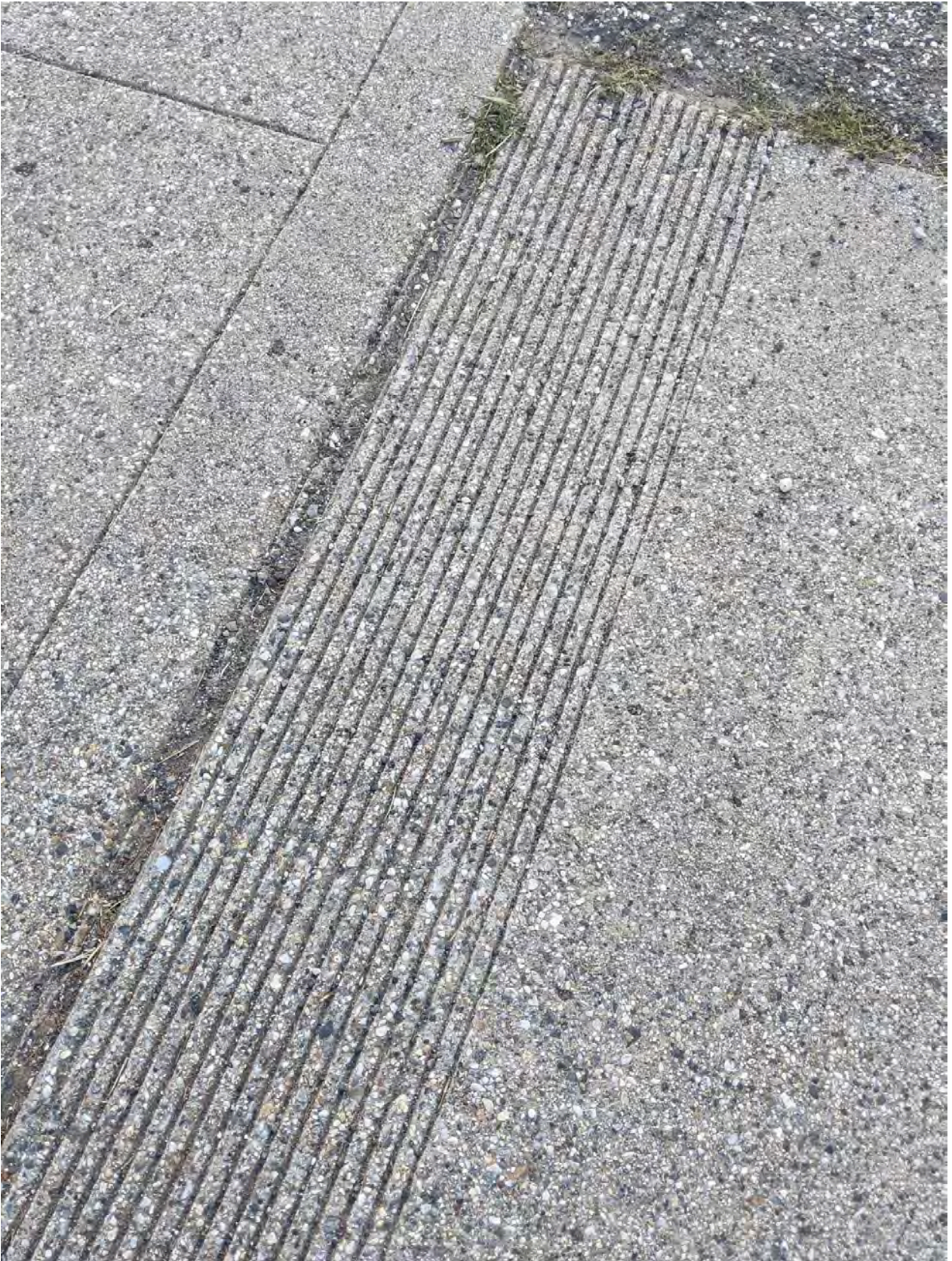
Figure 17 June Design Charette – Image of Non-ADA-Compliant Curb Ramp
